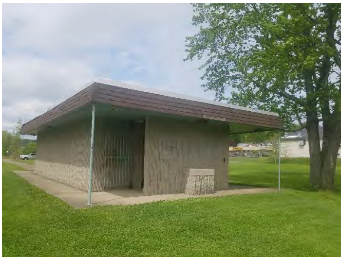
Restroom facility improvements badly needed at Chadakoin Park.
